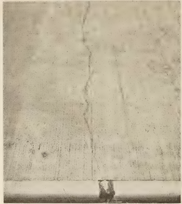
FIGURE 20.—TYPICAL CRACK IN A HEAVILY REINFORCED SECTION.
